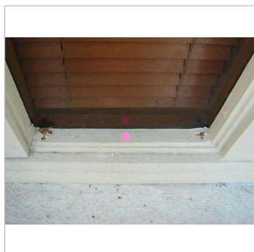
Figure 4J - damaged window trim at right of front entry
