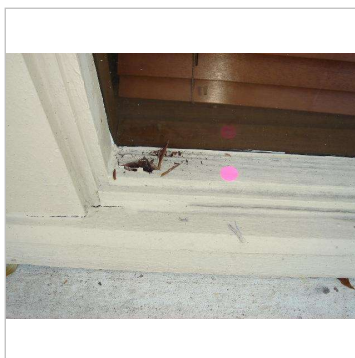
Figure 4K - damaged window trim at left of front entry
