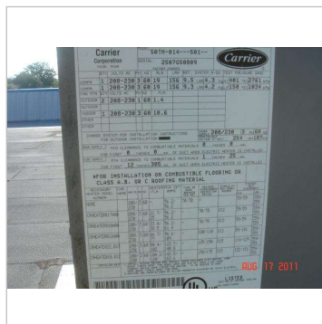
Figure 12B - Data tag on roof top unit
