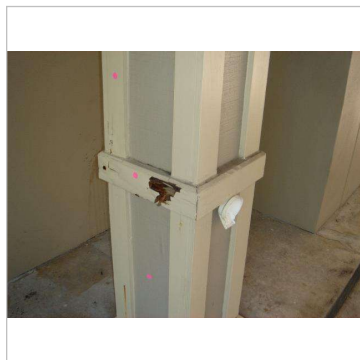
Figure 2A - damaged trim and siding on rear post due to sprinkler overspray
