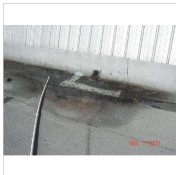
Figure 5A - Ponding water and repairs to seam at west side scupper
