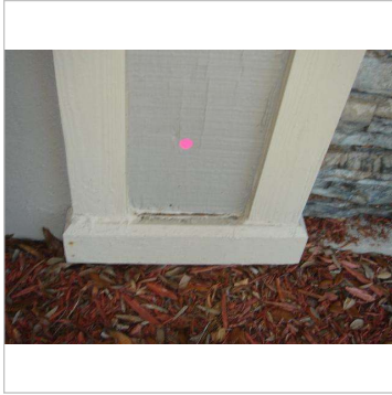
Figure 4A - damaged siding to right of front entry
