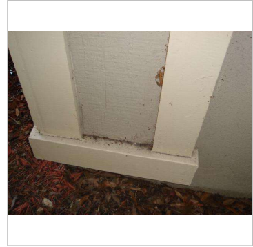
Figure 4C - damaged trim and siding on right side wall at front right corner
