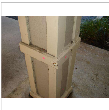
Figure 4G - damaged trim and siding on rear post
