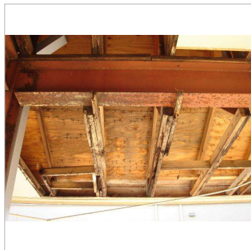
Figure 19A - damaged roof framing above drive thru
