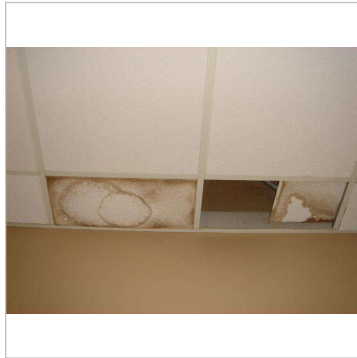
Figure 16A - stains and missing ceiling tiles in hallway to the break room and bathrooms
