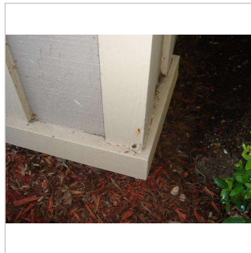
Figure 4E - damaged trim on front right corner
