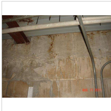
Figure 8A - minor corrosion to truss end and metal roof deck noted
