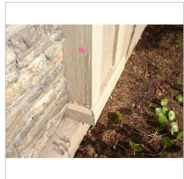
Figure 4F - damaged trim on left side wall
