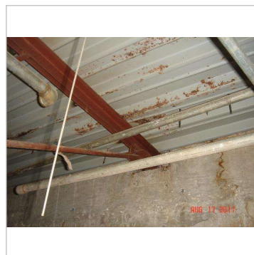
Figure 5F - Underlying roof deck-note corrosion and minor damage
