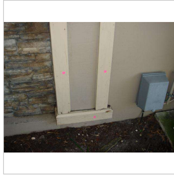
Figure 4B - damaged trim and siding on right side wall-2
