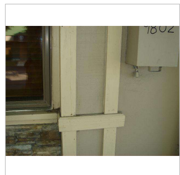
Figure 4I - damaged trim on right side wall at left of electrical room
