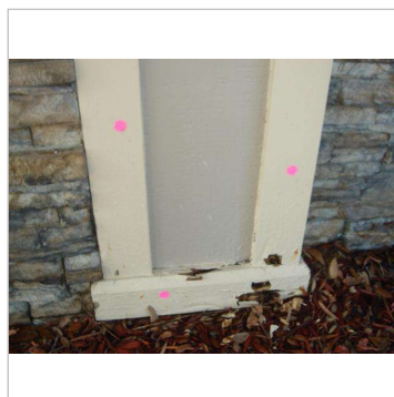
Figure 4H - damaged trim on front wall left of front entry
