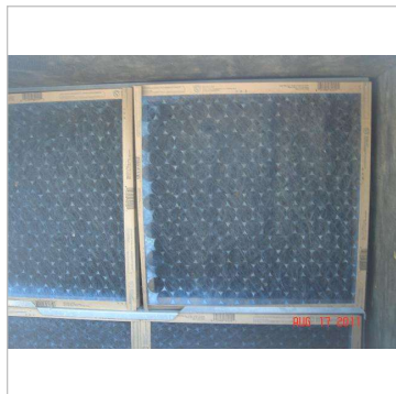
Figure 13A - Filters located under a panel in the roof top unit
