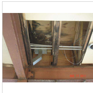
Figure 19C - damaged roof deck and underlying wood trusses
