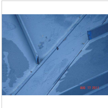
Figure 6A - caps missing on standing seam in rear valley
