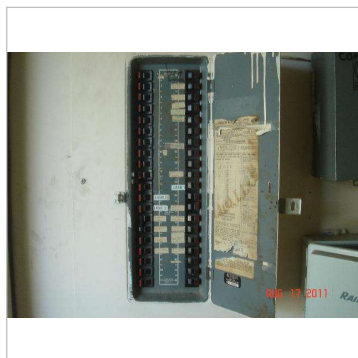
Figure 10A - Federal Pacific type sub panel
