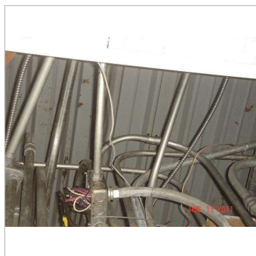
Figure 9A - Open junction box
