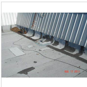
Figure 5E - mastic patch on seams up parapet wall and roof surface
