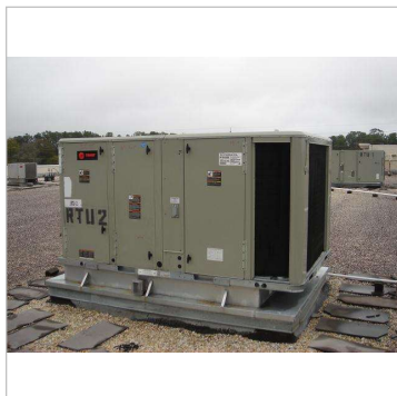
Figure 21D - rtu 2 10ton
