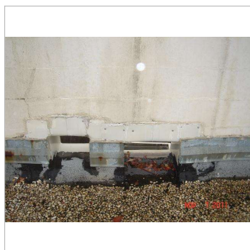
Figure 12A - Scuppers at rear appear to have been sealed and re-flashed
