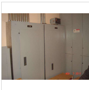
Figure 19D - Sub panels with surge protector
