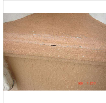
Figure 7C - cracks in column base stucco banding
