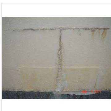
Figure 13D - cracks and efflorescence in block parapet wall
