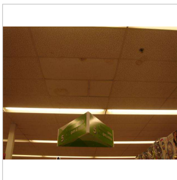
Figure 11B - dry stains on ceiling tiles over aisle #5
