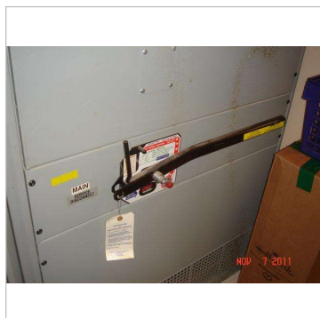
Figure 17A - Main service disconnect
