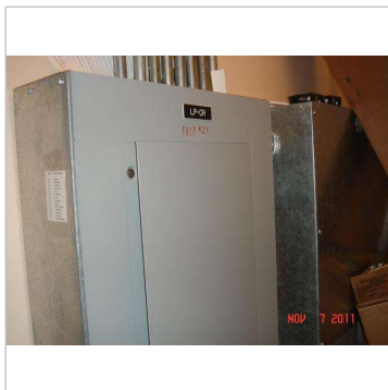
Figure 19B - sub panel
