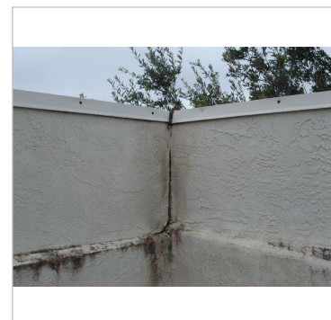
Figure 6I - cracks at facade wall intersections
