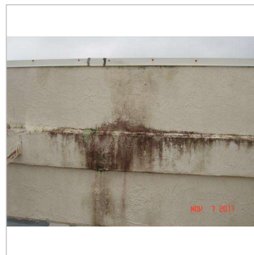
Figure 13C - stains and cracks in stucco on facade wall
