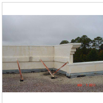
Figure 6H - water ponding on roof at west side facade
