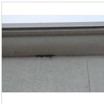
Figure 13A - Evidence of leakage on parapet wall at left side
