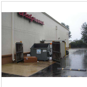
Figure 3A - enclosure at rear
