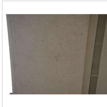
Figure 6E - cracks in stucco-stains on soffit at front-2
