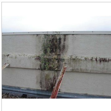
Figure 13B - stains on facade-1
