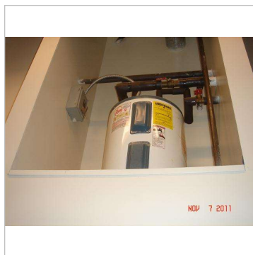
Figure 20A - water heater for bathroom and employee kitchen area
