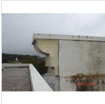
Figure 7A - decorative banding is damaged-foam is showing in this photo
