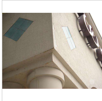
Figure 7B - corrosion and stains on stucco walls and stucco bands at front left corner
