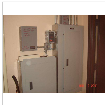
Figure 19C - outdoor lighting panels and surge protector
