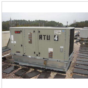
Figure 21B - rtu-4 4ton
