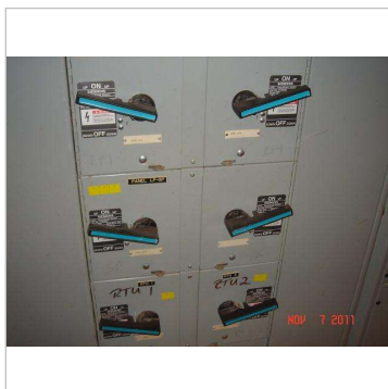
Figure 17B - Main switching center bottom half
