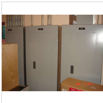
Figure 19A - Sub panels adjacent to the main panel
