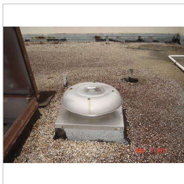
Figure 22A - roof top portion of ventilation system
