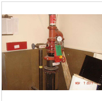
Figure 23A - fire system riser
