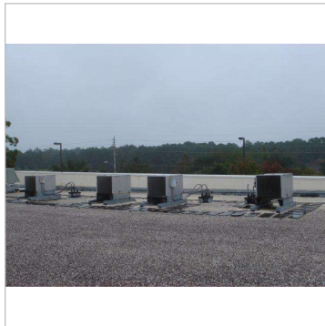
Figure 25A - 4 compressor units for in-store coolers
