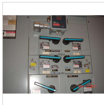
Figure 17C - Main switching center
